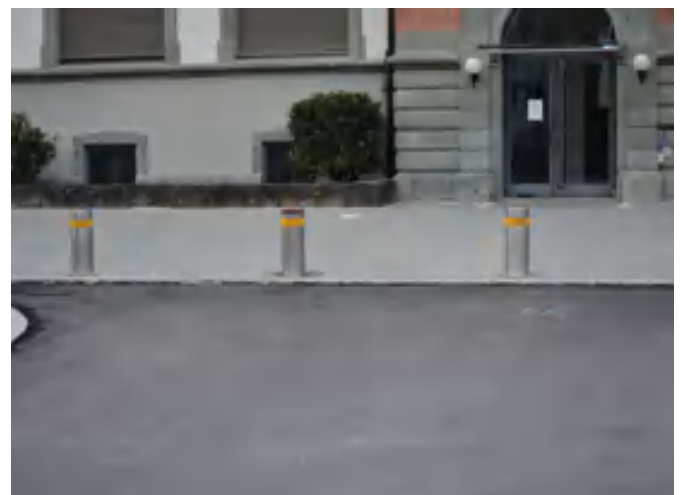
Fixed bollards and Retractable bollard school Thal
