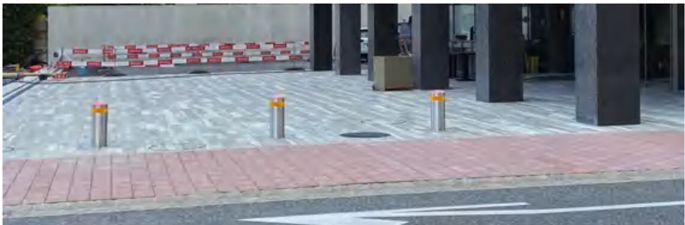
3× Borne escamotable 2, bâtiment commercial
